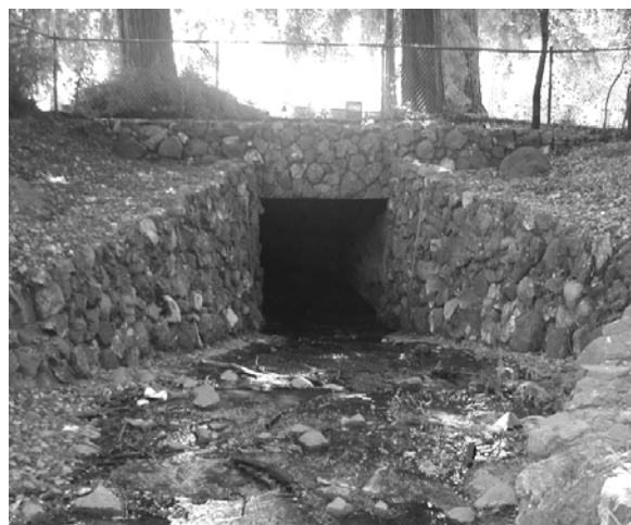
Single box culvert on Strawberry Creek at Shattuck Avenue in Berkeley, CA.
